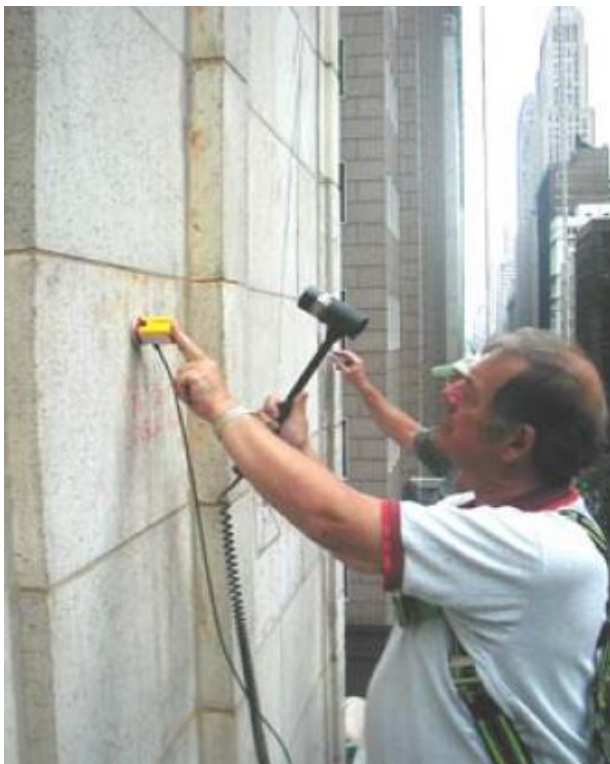
Implementation of s'MASH Impulse Response for detection of terracotta panels cracking, Chicago, USA
