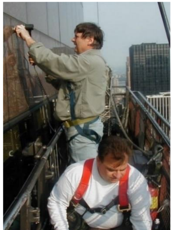
Implementation of s'MASH Impulse Response for detection of lack of anchoring of granite panels, New York, USA
