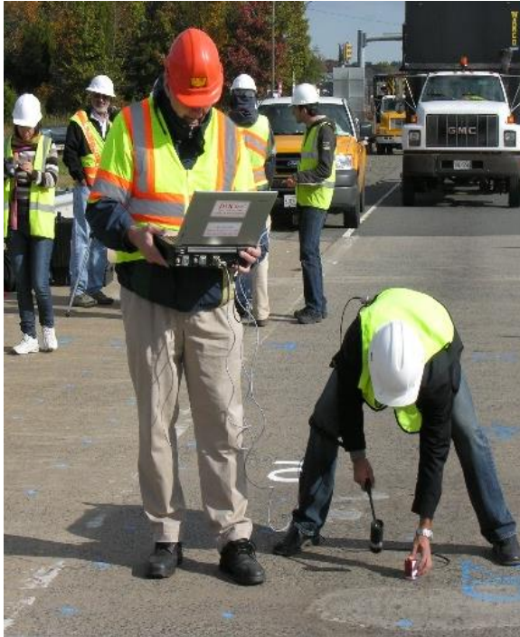
Implementation of s'MASH Impulse Response on bridge deck for defects, West-Virginia, USA
