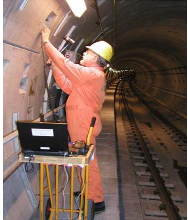
Implementation of s'MASH Impulse Response on tunnel for voids in the injection behind the tunnel elements, Denmark
