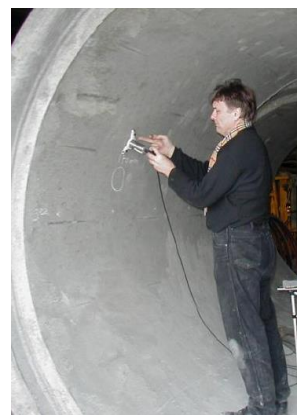
Sewer tubes, Denmark Delaminations
