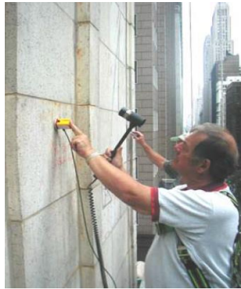
Terracotta Panels, Chicago Cracking / debonding
