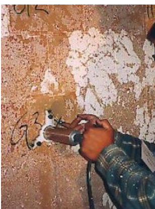
Pulp Plant, Canada De-bonding of tiles
