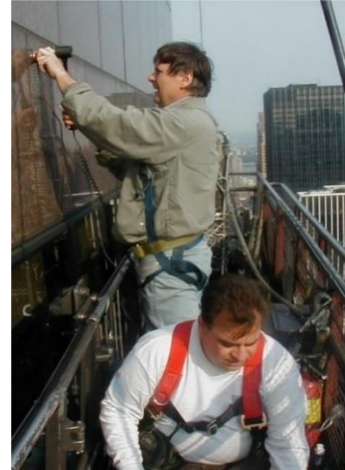
Granite Panels, New York Missing anchoring
