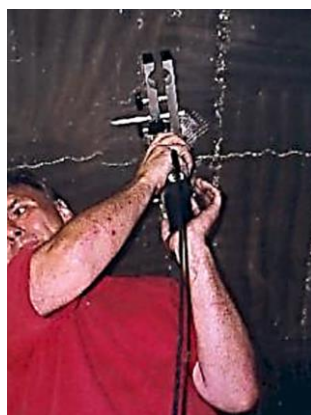
Fire damaged ceiling, Germany Depth of cracks
