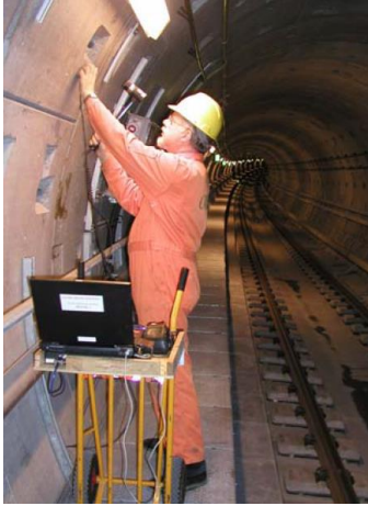
Tunnel lining, Denmark Voids in injection
