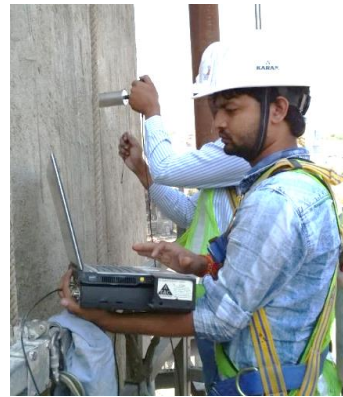
Avantech team carrying out Impact Echo test on wall of silo using the DOCTer Impact Echo Test System
