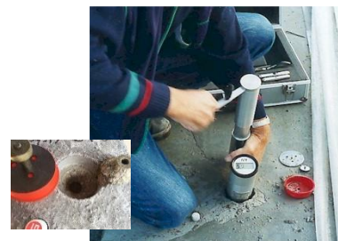
Garage parking structure, UK Covered by heavy plastic sheet and wet mats. Pullout matched the lab strength
