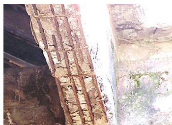
Severe cases of carbonation damage
