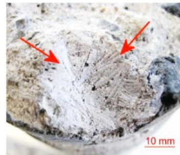
2. Ice flowers formed between aggregates and cement paste before hardening of the concrete (sign of early frost exposure).
