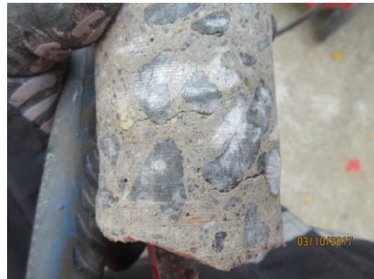
Core B. Intact but with cracks around the aggregates and reinforcement.
