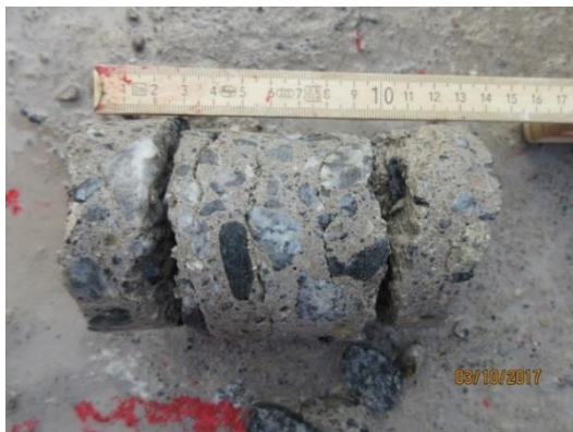
Core C. Delaminated. Typical ASR-cracks.
