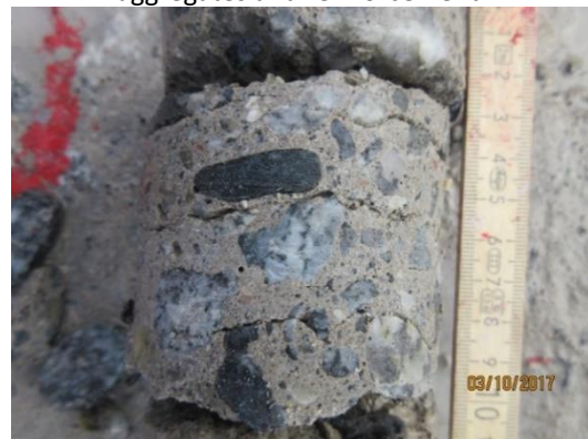
Core C. Delaminated. Typical ASR-cracks
