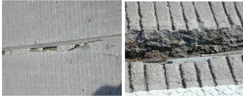
Example of Freeze and Thaw cracking of the longitudinal joints of a concrete highway due to an improper air-void system in the presence of wet (saturated) concrete and freeze-thaw cycles.
